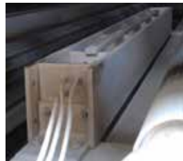
ST-3300 in a high-temperature application.
